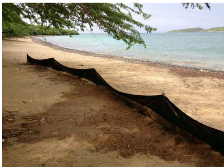
Figure 21. Silt fence at the Tamarindo restoration holding back sediment from nearshore waters from an upland dirt parking lot and restoration project
