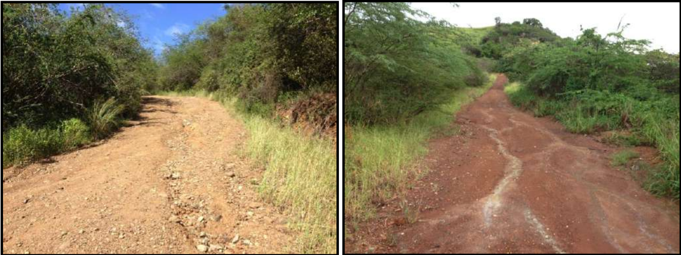
Figure 18. Dirt roads as a source of sediment (note the surface runoff over the roads creating erosion and resulting in fine sediment losses)
