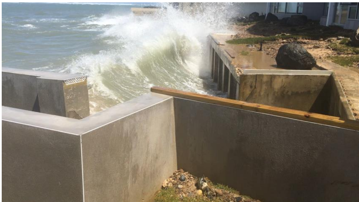
Figure 21. Unprotected vertical seawall in San Juan Puerto Rico.
