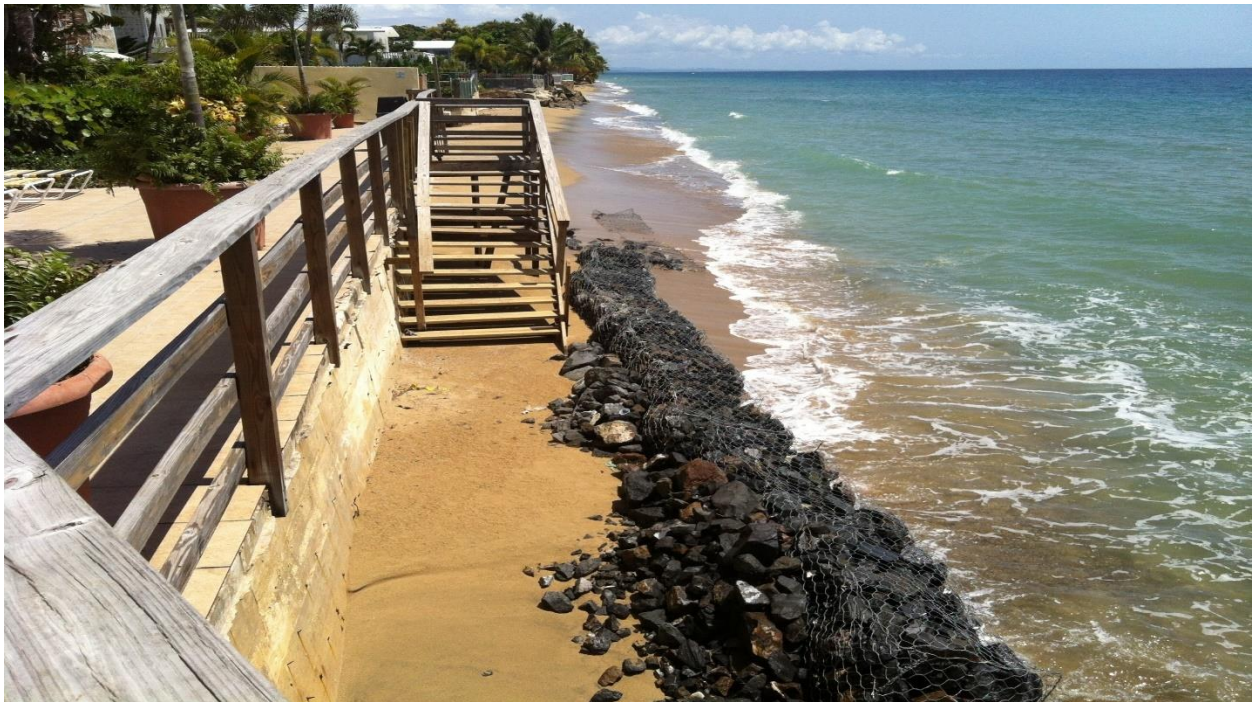
Figure 10. Failed gabions along shoreline in Córcega, Rincón. Wire cage mesh has broken open, posing safety threat, and releasing rocks onto beach.
