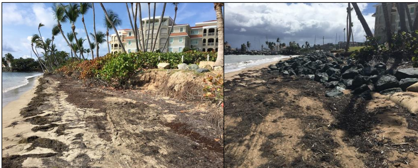
Figure 22. (Left photo) Eroding shoreline prior to bank stabilization at Palmas del Mar. (Right photo) Development of Plaza del Mar revetment, Palmas del Mar
