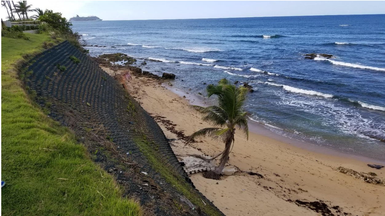
Figure 13. Synthetic gabions for San Juan Bluff Stabilization Project in Old San Juan, Puerto Rico. Photo taken on October 25, 2018.
