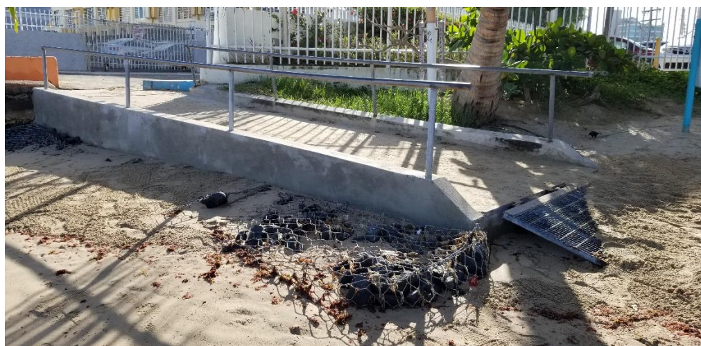
Figure 12. Gabions used as coastal protection for walkway in Punta Isla Verde, San Juan, Puerto Rico. Top photo taken on September 21, 2018 and bottom photo taken on October 25, 2018.
