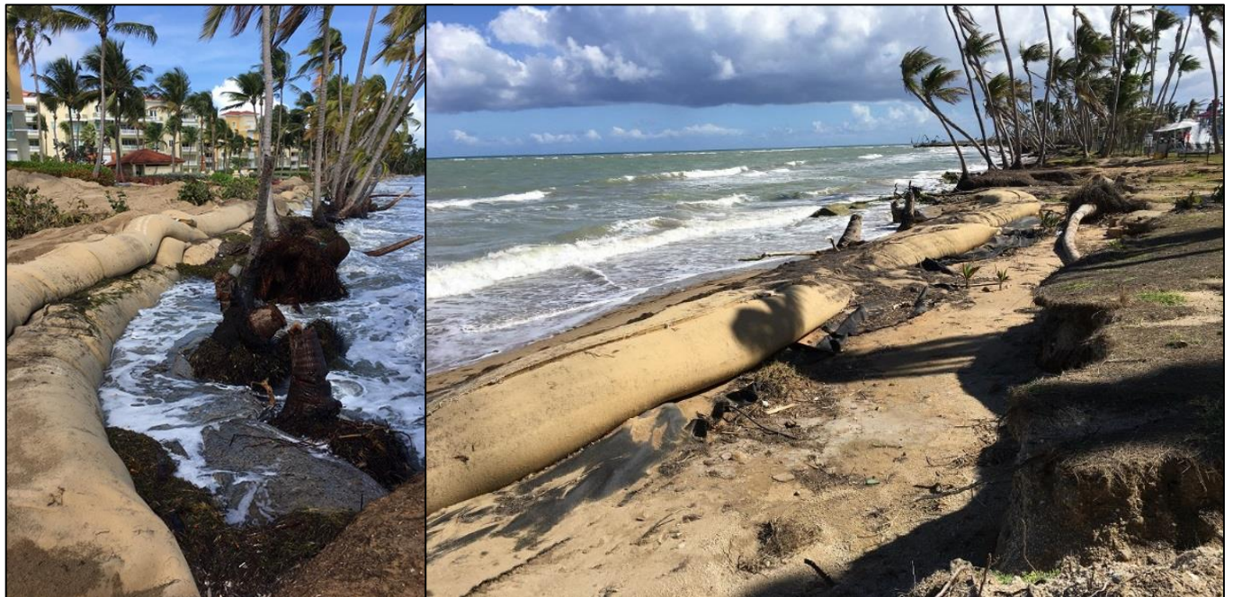
Figure 19. Erosion of the shoreline around geobags at Marbella Club, Palmas del Mar in December 2016, approximately 1 year after construction (left photo). Erosion around geobags at Marbella Club after Hurricane Maria (right photo).
