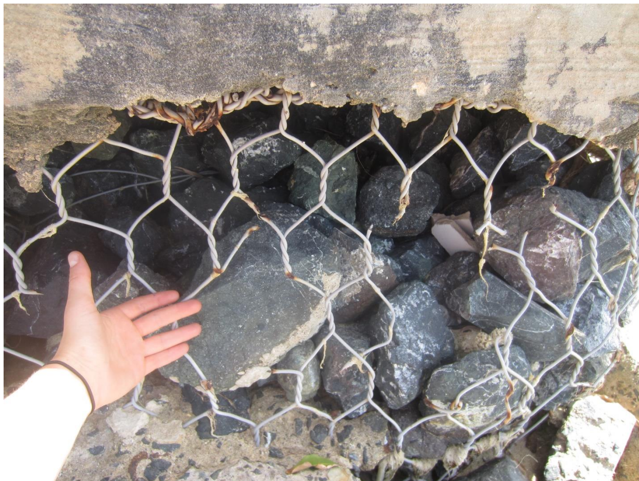
Figure 11. Broken wire mesh of gabions used as foundation material for concrete walkway at Punta Isla Verde, San Juan. Photo taken September 21, 2018.
